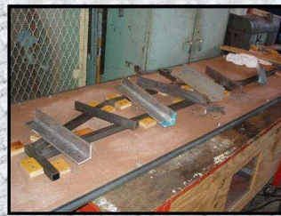
Individual Frame Rails were place on the jig table and secured with wooden blocks. This method insured frame rails would be identical once taken out of the jig.
