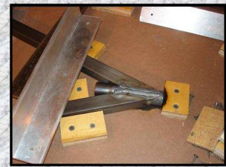
Weld areas were properly prepared, before laying down weld material. Corners were machined for proper fit-up, and steel was cleaned with Acetone to remove contaminants.
